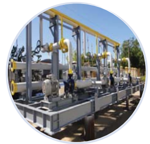
Pre-Packaged Pump Skid
